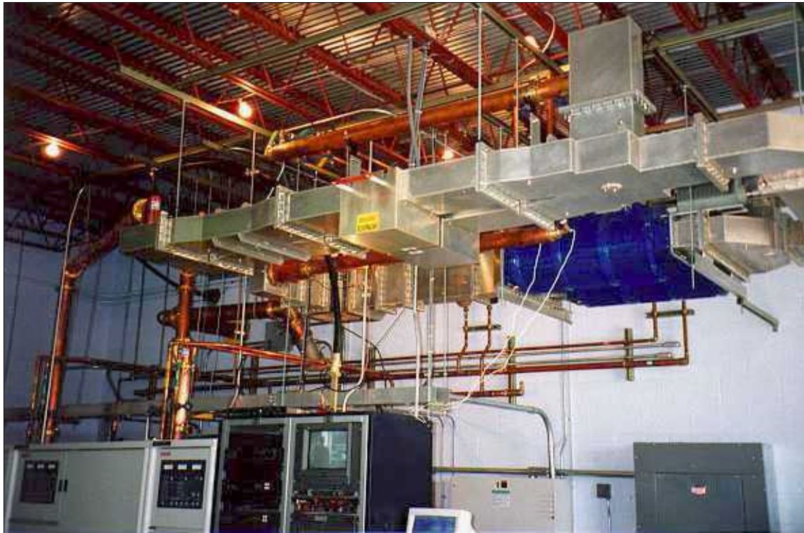
Figure 2. Photo, IOT ceiling-mounted RF system lower left: IOT amplifier cabinets and PIE racks foreground: WR1500 waveguide magic tee combiner w/ water column coaxial RF loads background: high power output bandpass filter (blue cavities) background: cooling system pipes along back wall lower background: line control cabinet against wall (just behind PC screen)
