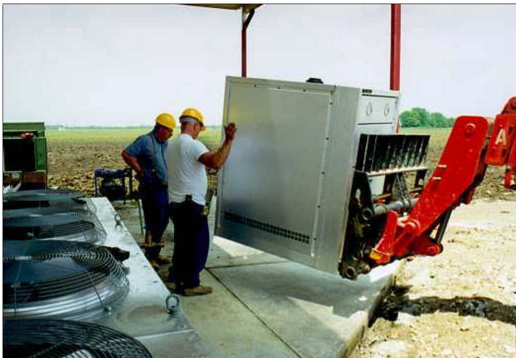
Figure 4b. Photo, IOT system outdoor components: workers move pump module into final position.
