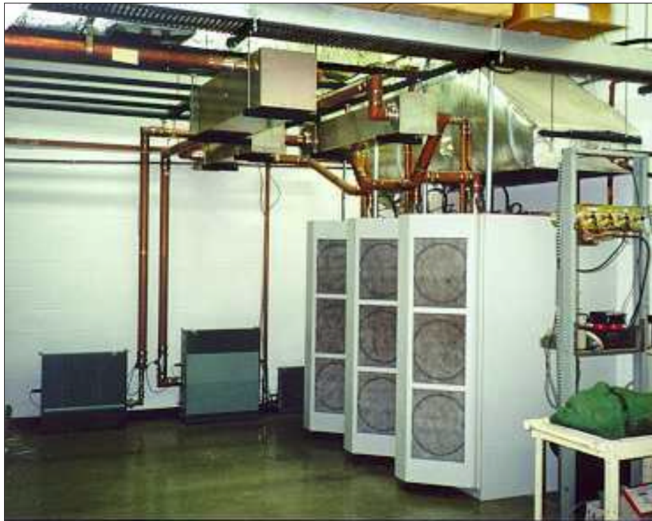
Figure 5. Photo, solid-state VHF transmitter installation right: rear view of three PA cabinets showing air intake filters right top: air exhaust manifold above transmitter cabinets (silver duct) center top: RF system with 3 1/8 inch rigid coaxial line background: reject loads for 3 dB power combiners on floor note: output bandpass filter not shown in picture note: room air input plenum not shown in picture
