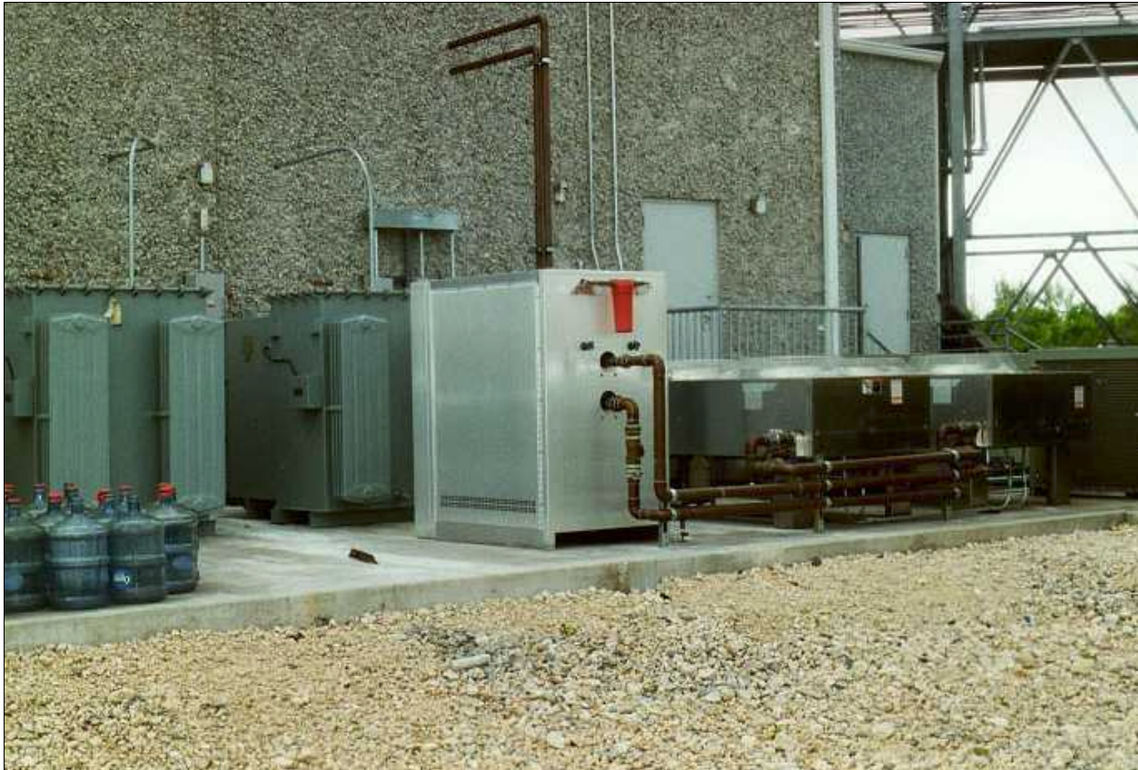
Figure 3. Photo, IOT system outdoor components.
